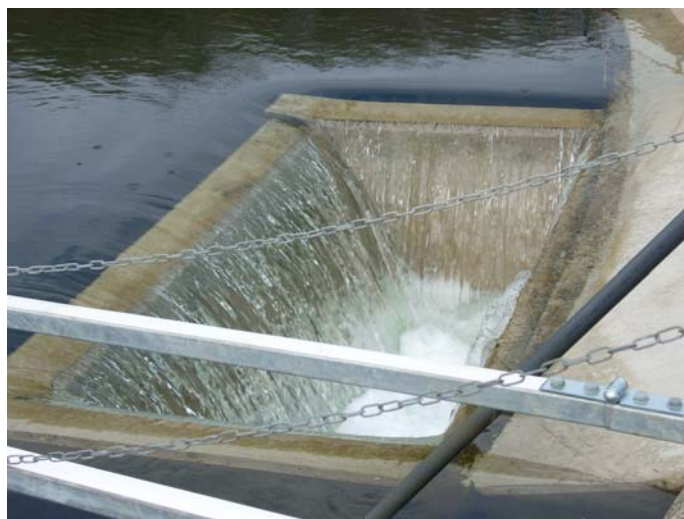
Figure 18: Final effluent from sewage treatment being discharged to the watercourse.
