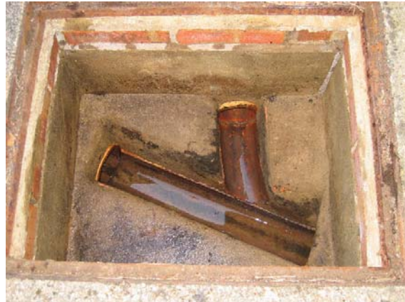
Typical inspection chamber
