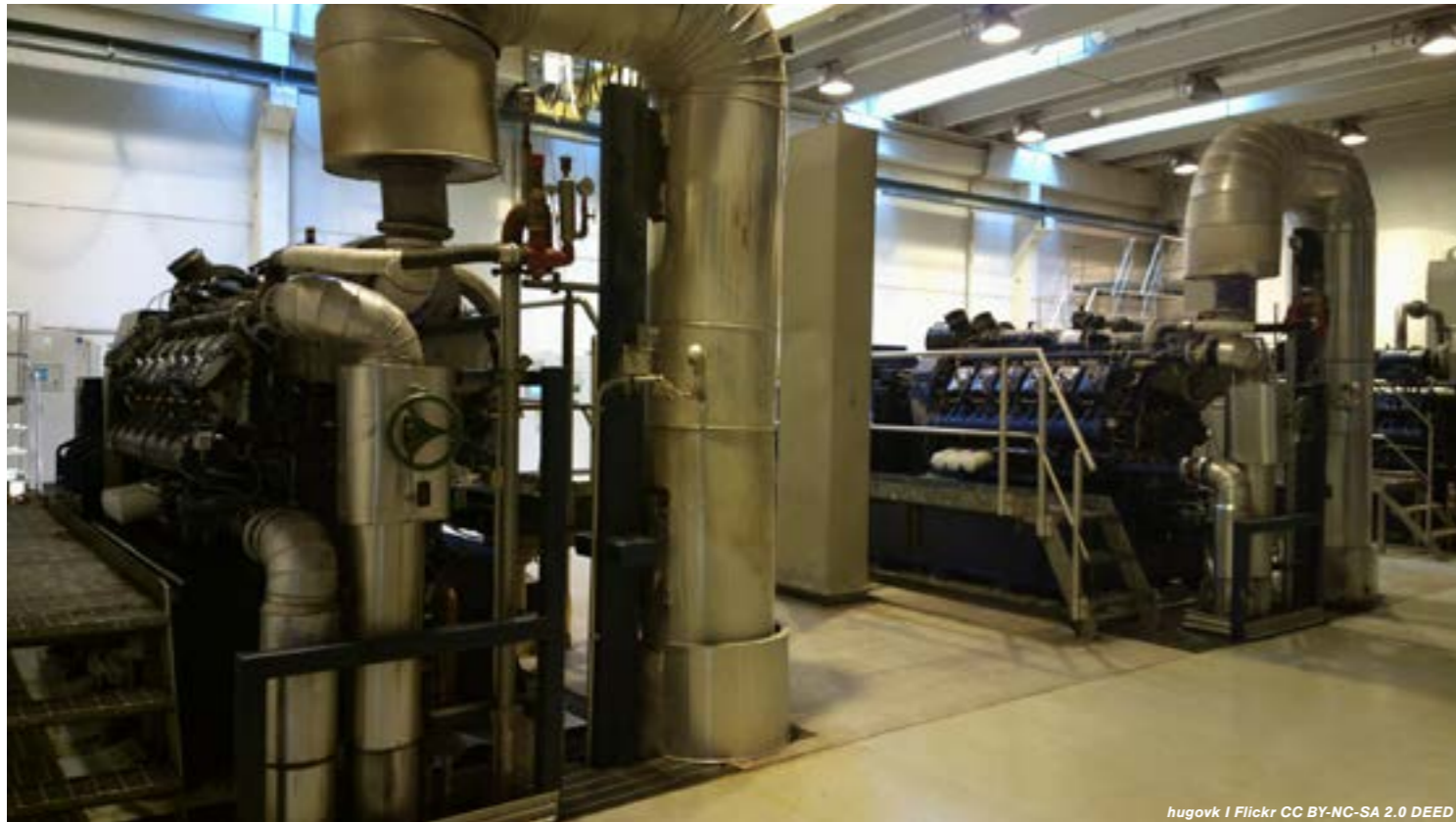
Generating electricity from biogas at the HSY Viikinmäki waste-water processing plant
